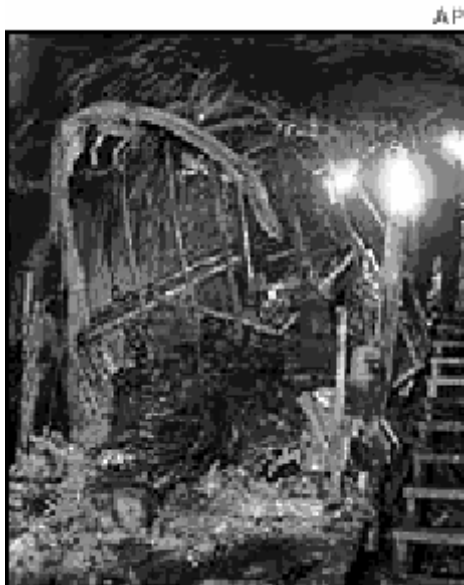
Picture 2. Interior of the tunnel after fire (1)
